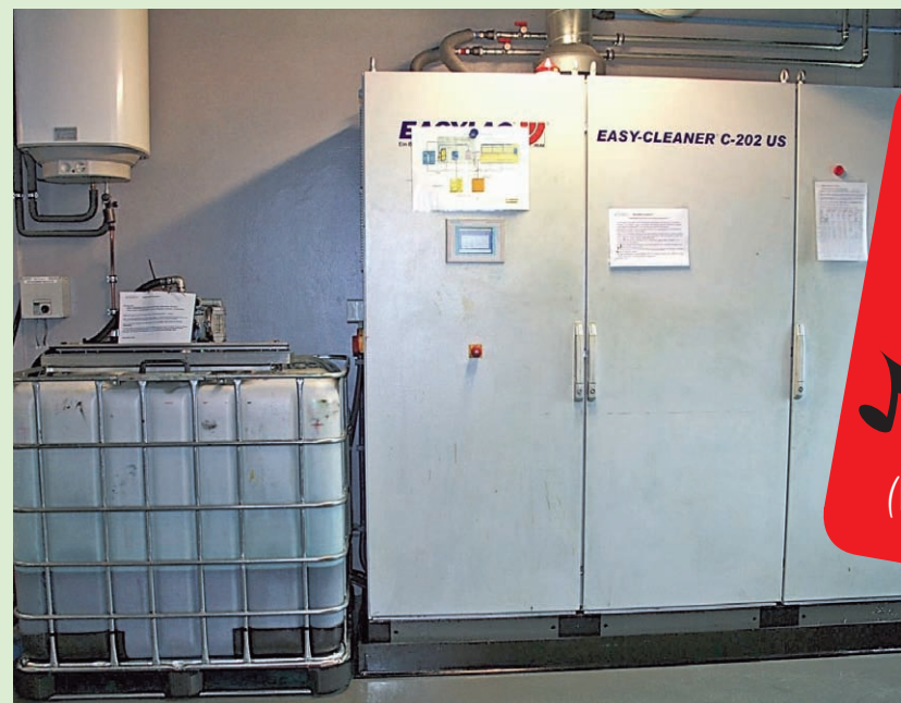
The automatic cleaning system in Best
